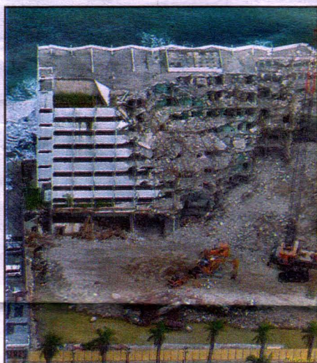
One of Toledo Engineering's demolition projects in the Condado Beach Trio area
